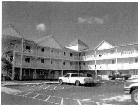
Figure 14-29. Elevated external walkways such as this are not allowed.
